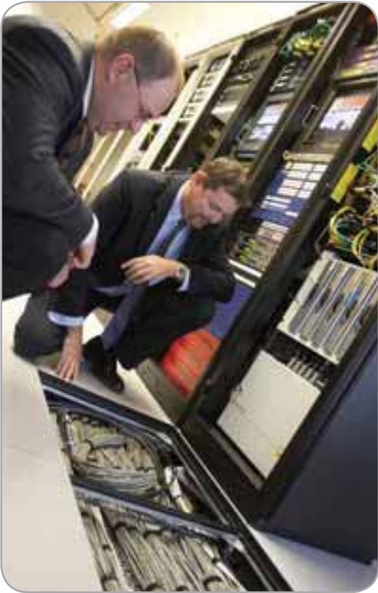
Heath Mackey, High Court and Grant Bawden, Intravision examine the under-floor cabling.
